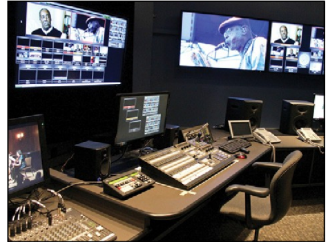
One of the two Granite 5000 systems installed at WHYY-TV
